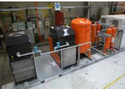
Compressor system consisting of (left to right) a nitrogen generator used for food packaging, four air filters, a receiver tank and two compressors.
