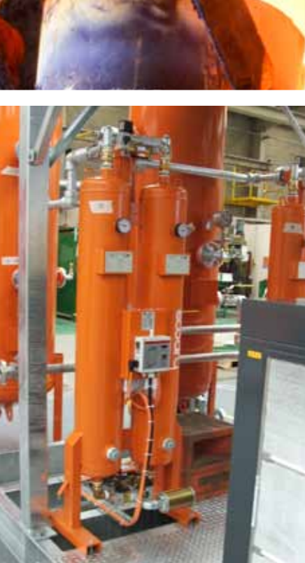
Air compressor filters should be kept clean to reduce pressure drops.
