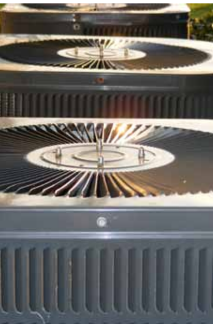
Audits of existing air conditioning systems can help to identify efficiency opportunities.
