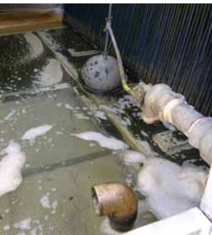
Check the make-up ball float and valve are performing at the optimum level to reduce unnecessary blow down.
