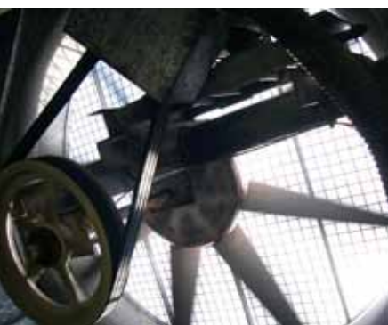
Installing a variable speed drive on the fan to reduce drift and save energy.
