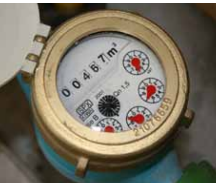
Water meters should be installed on all process equipment that uses a significant amount of water.
