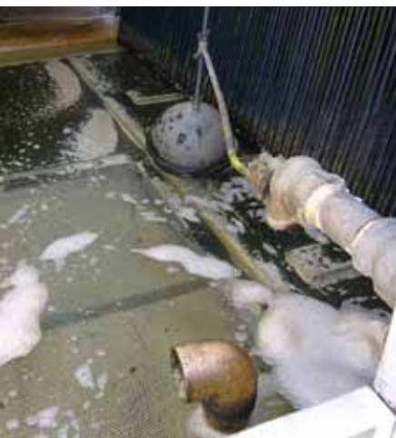
Check the make-up ball float and valve are performing at the optimum level to reduce unnecessary blow down.
