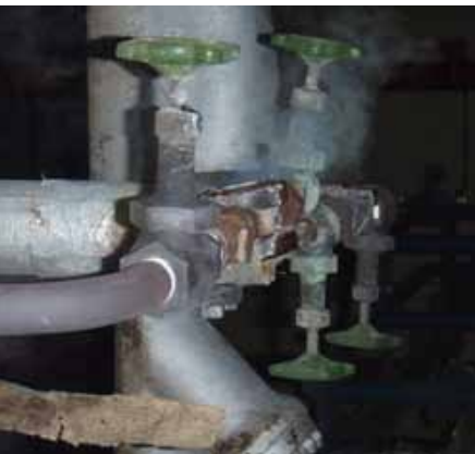
Repair steam leaks promptly to reduce energy loss.
