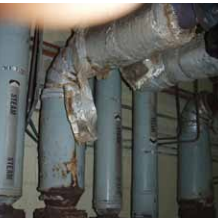
Deteriorated insulation allows heat loss so repair promptly
