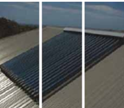
Evacuator tube collector
