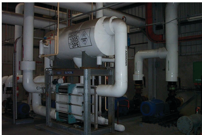
The compressor, evaporator and condenser should suit the refrigeration duty.
