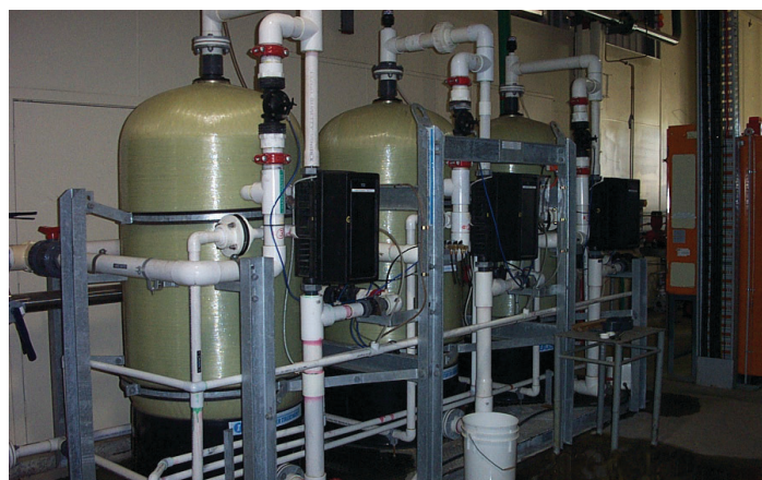
The treatment of boiler feedwater will help to minimise scale build-up, which acts as an insulator and inhibits heat transfer.
