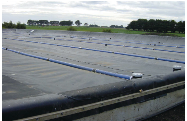
Anaerobic digester with cover for biogas capture — Warrnambool Cheese and Butter, Allansford
