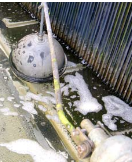
Regularly check level of cooling tower
