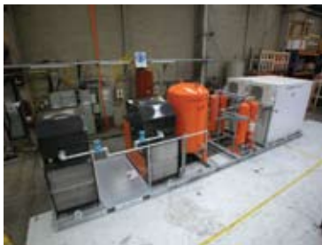
Compressor system consisting of (left to right) a nitrogen generator used for food packaging, four air filters, a receiver tank and two compressors.
