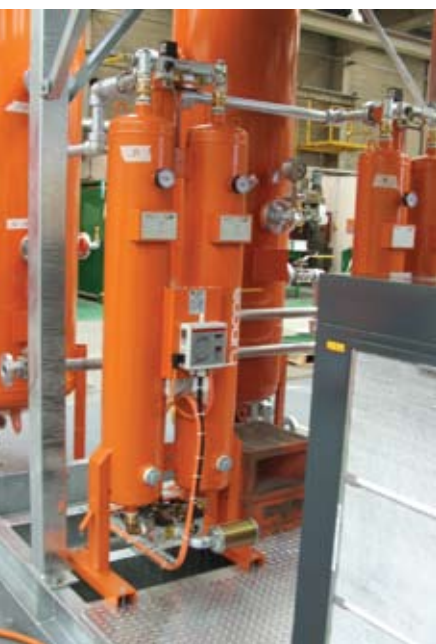
Air compressor filters
