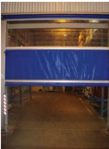
Self-closing doors and strip curtains can be used to minimise heat ingress to refrigerated areas.
