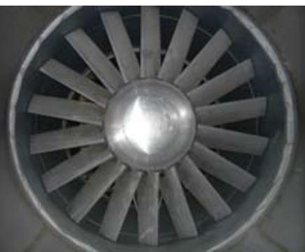
Operating fans only when required will reduce energy consumption.
