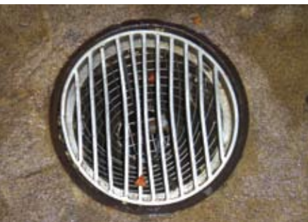
Strainers on drains can reduce waste entering wastewater system
