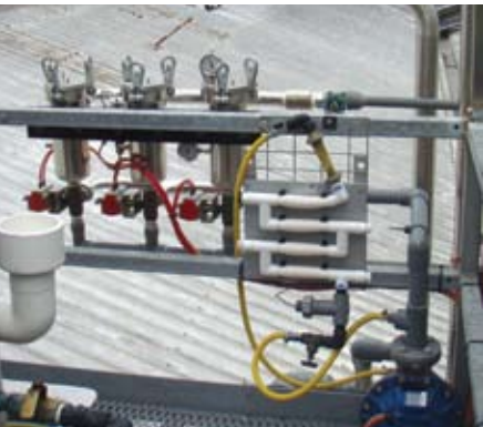
Golden Circle hydrocavitation filtration system.
