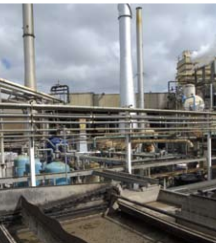
DAF treatment system is useful in removing FOG
