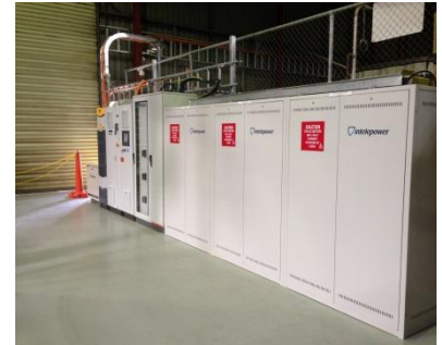
Battery Energy Storage System (BESS)
