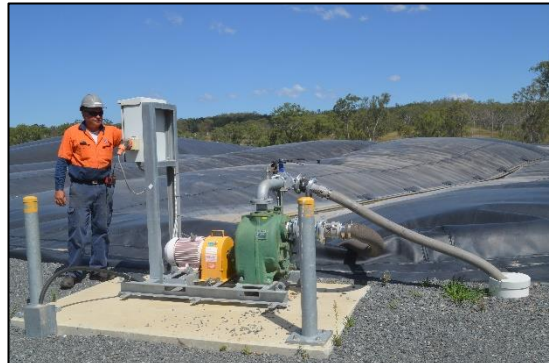
Turning on stormwater pump Image: Teys, Beenleigh
