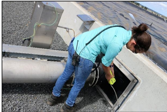
Checking for leaks in the CAL wall Image: NB Foods, Oakey
