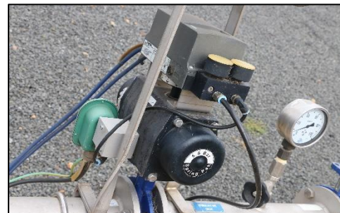
Shut off system Image: NB Foods, Oakey
