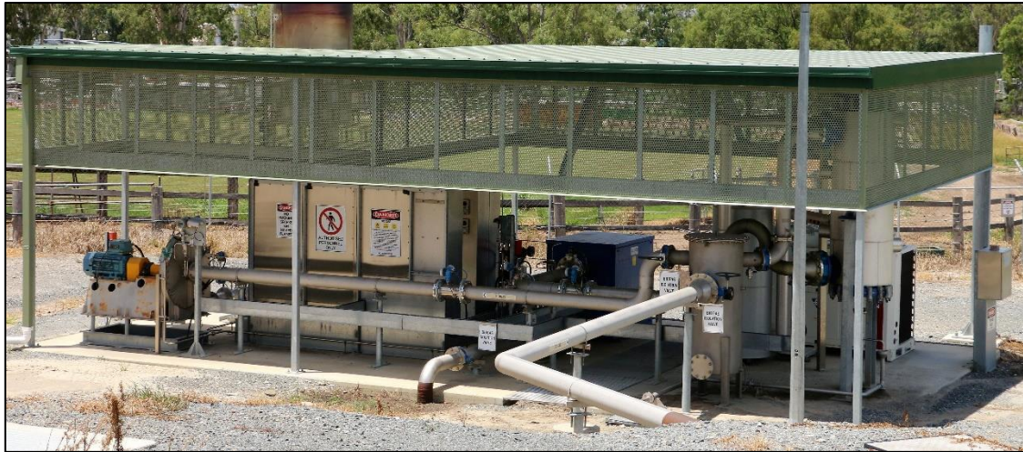
Pipeline from CAL delivering biogas: Stainless steel knockout pot(right) to blower (left)
