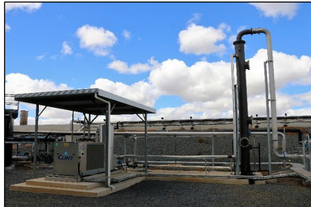
Stripping tower and dehumidifier
