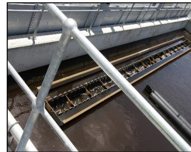
Clarifier weir Image: Teys, Beenleigh
